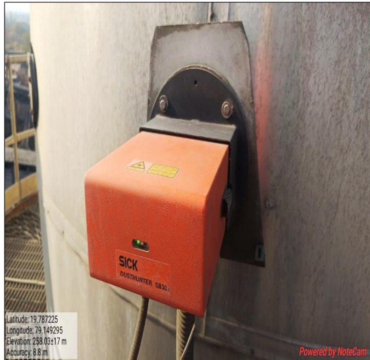
CEMS Installed at Stack
