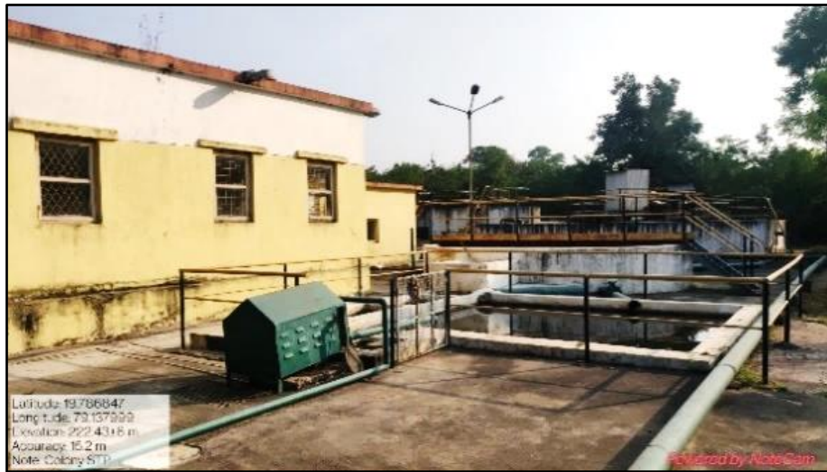
Sewage Treatment Plant at Colony
