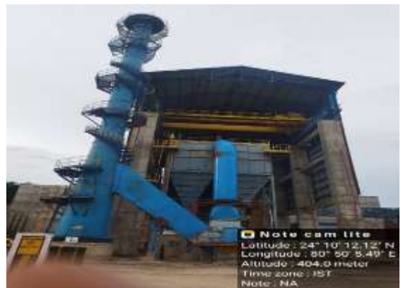
Adequate Dust Collectors at
