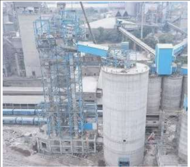
Fly ash Unloading Pit
