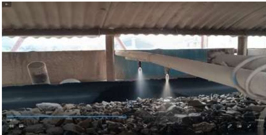
Water Spray at Lime stone Belt conveyor
