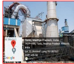
Line-2 Cooler ESP
