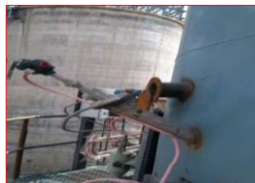
Opacity Meter CM BH Stack-2
