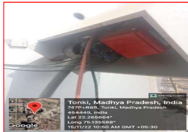
Opacity Meter (PM) L-2 Cooler ESP Stack
