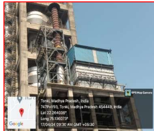
Line-2 Coal Mill Baghouse
