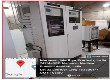
L-2 Sox & NOx Analyzer RMBH Stack
