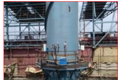
Opacity Meter CM BH Stack-1
