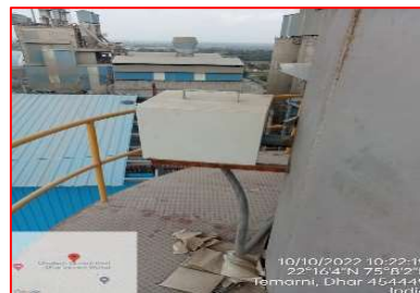
Opacity Meter CM BH Stack-3
