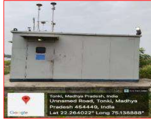
CAAQMS-2 Near Power Switch Yard
