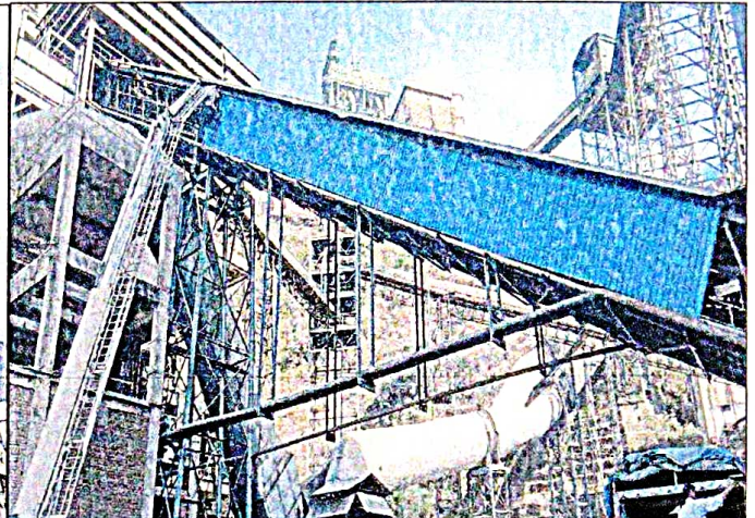
Covered Conveyor belt
