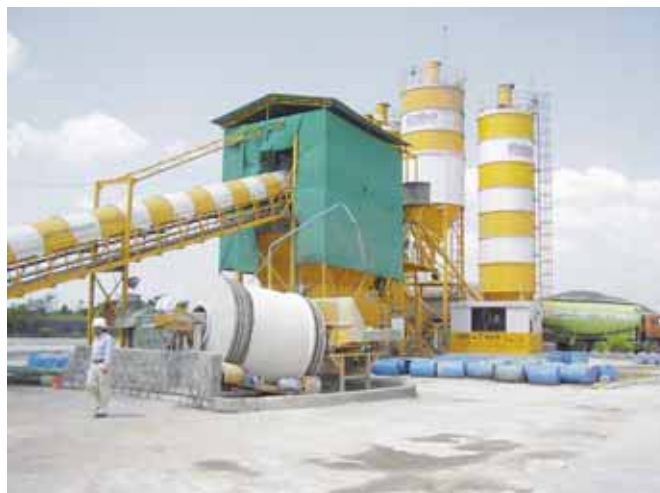
Ready Mix Concrete Plant
