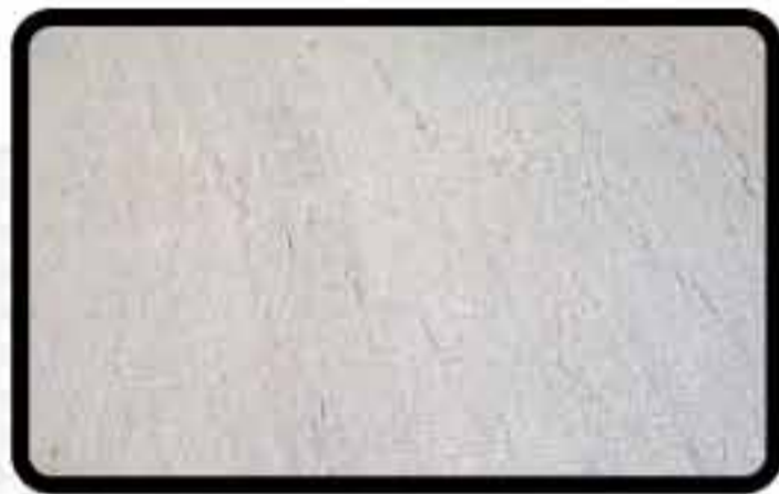
Plastic Shrinkage Cracks
