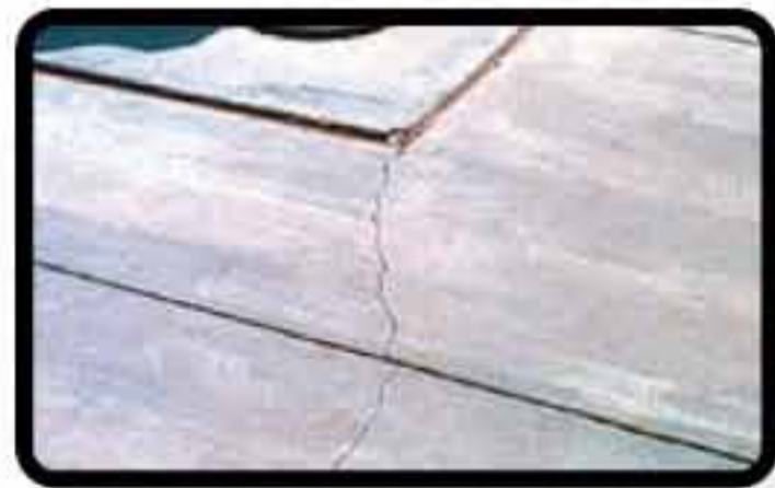
Drying Shrinkage Cracks
