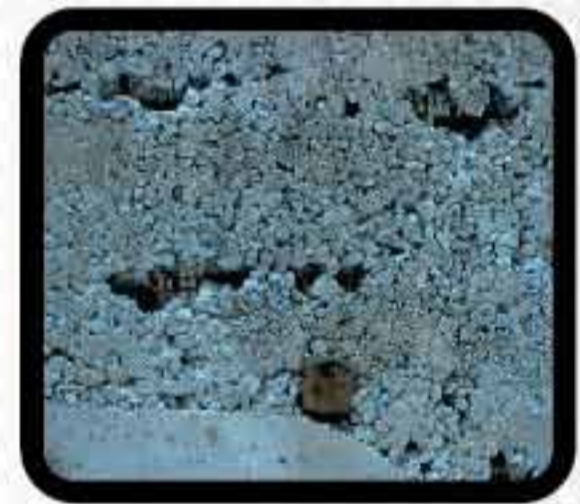
Formation of Honey Comb Due to Improper Compaction.
